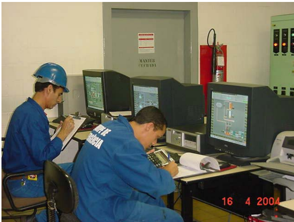
Petrom engineers monitor and operate three reactors from operator stations networked via PROFIBUS to both field instrumentation and discrete I/O, greatly simplifying remote configuration and diagnostics.
