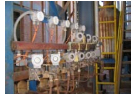
Figure 8: Field equipment connected to the PROFIBUS PA network configuration screen
