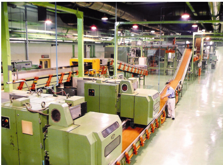
Rather Than Hard-Coded Communication, Xuzhou Tobacco Factory in China Configures Flexible Data Exchanges Between Controllers With Profinet CBA
