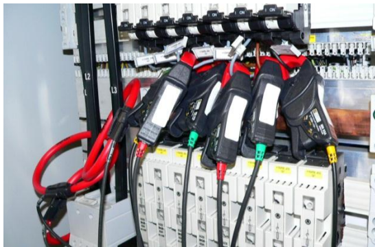
Figure 4 – Arrangement of current (I) transformers / flexible current transducers for high power ratings (background); and split-core transformers for lower power ratings (foreground)
