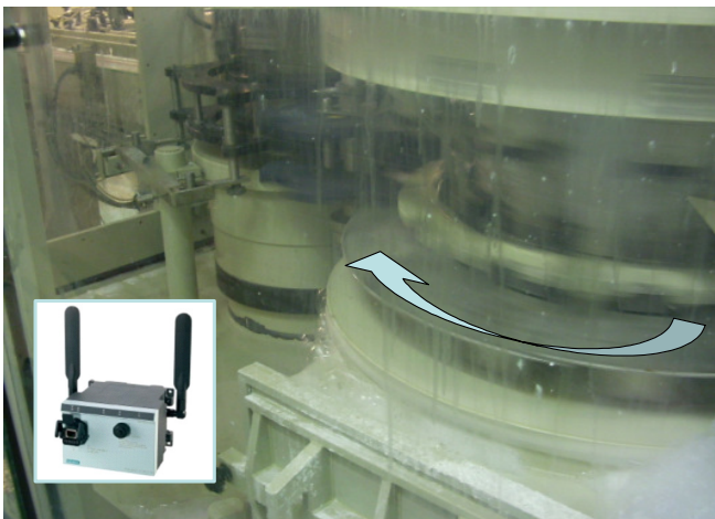
Using A Wireless Connection In Place Of Slip Rings Helped Improve The Reliability Of The Network Connection In HGI's Filling Machines
