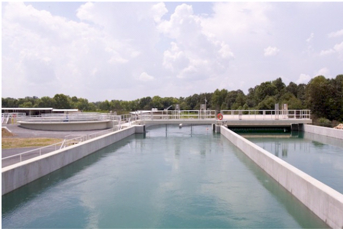
This Water Treatment Plant Uses Profinet Over A Fiber Optic Ring Topology To Network Controllers And Drives Separated By Long Distances
