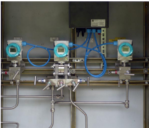
The Gas Compressor Station Uses Pressure Transmitters with SIL2 Safety Loop Capability. SIL3 Is Possible In A 2oo3 Configuration, as Shown Here.
